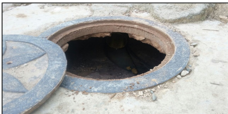
Figure 5 . Inspection well in poor condition.
