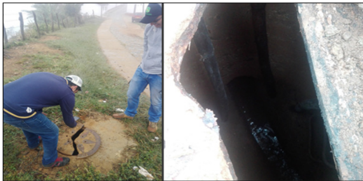
Figure 4 . Broken inspection of the well cover and internal state of the well.
