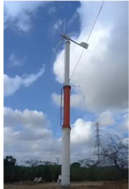
Figure 3. Aeolos-H 5 kW wind turbine Source: Authors' own photograph
